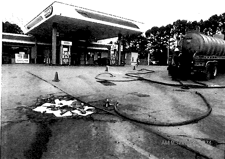
Close up of fuel/water evacuation process on February 2, 2024 adjacent to the seep.
